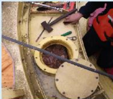
SBM main bearing grease Inspection
