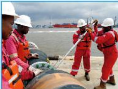
Floating Hose Connection
