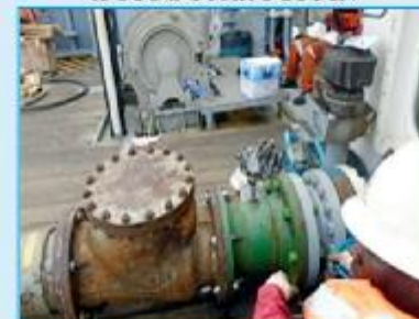
Crude Oil Back- Flushing From Hose Line With The Help Of Non Returned Valve
